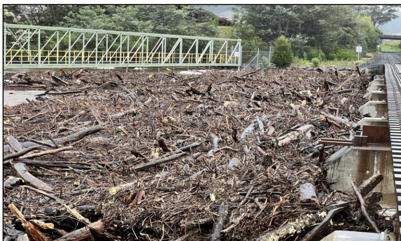
Debris accumulation at Railway Bridge in the October 2022 flood event (SES)
